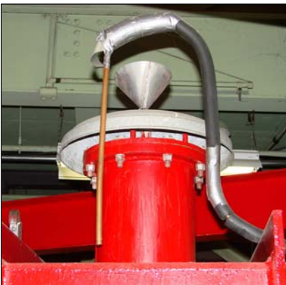
When the DP's are opened its time to fill the tank cold trap with liquid nitrogen. This trap is located on top of the DP valve chamber.
