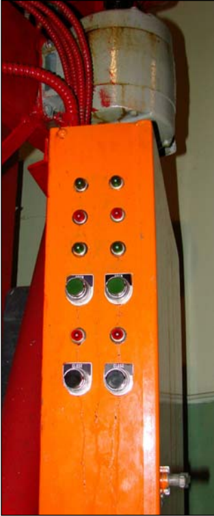
Opening DP main valves
