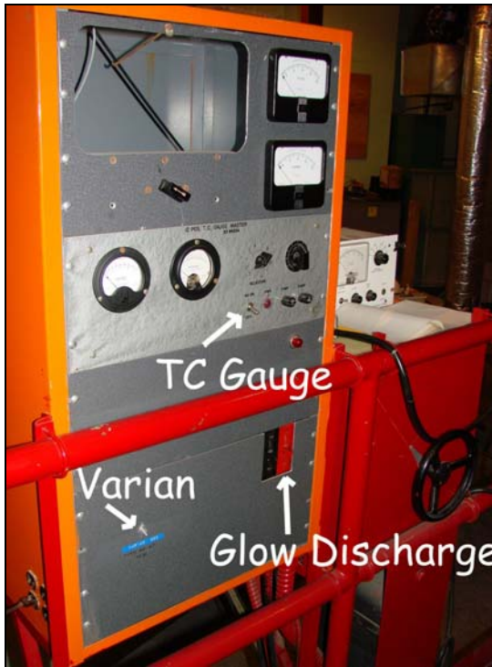
The Control Panel
